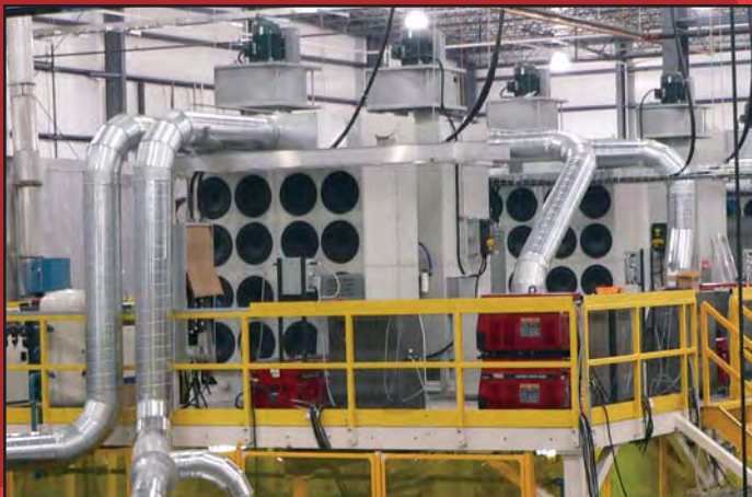
RP8-2 Collects Smoke/Fumes from Robotic Weld Cell
