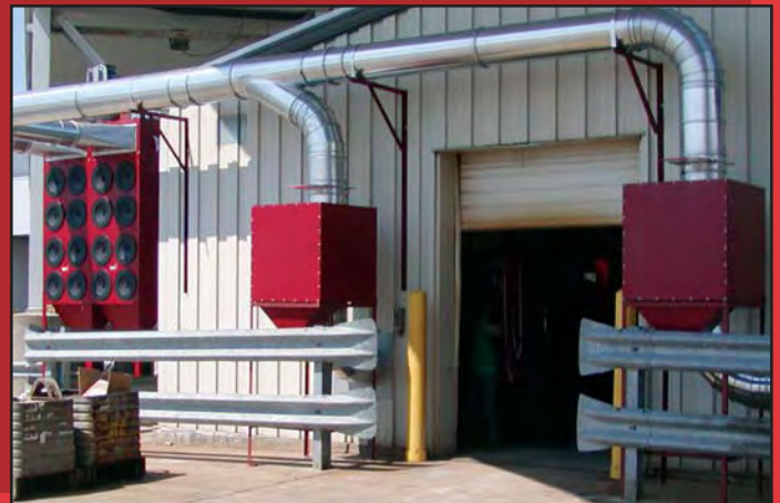
RP8-2 with spark arrestors collects laser smoke.
