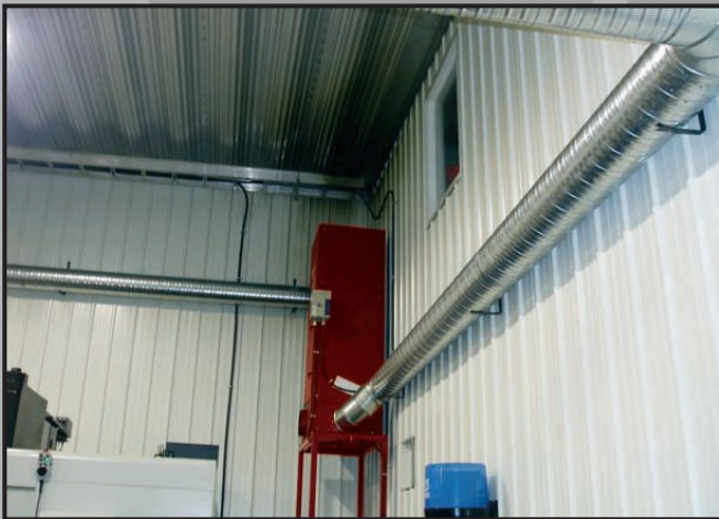
OM3510 on custom floor stand, ducted to CNC Milling Machine.
