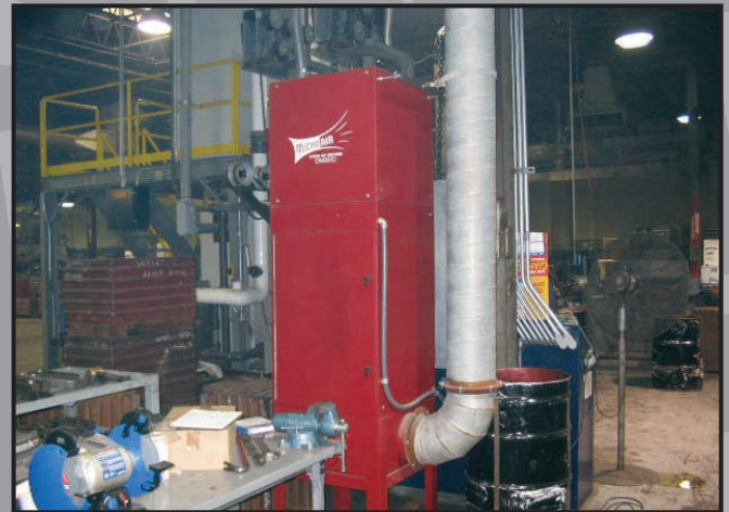
OM3510 ducted to lathe.
